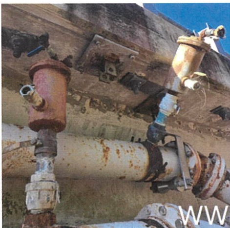
Figure 3: Air release valves with corroded fit-up points
