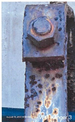
Figure 11: Pitting corrosion on pipe hangers
