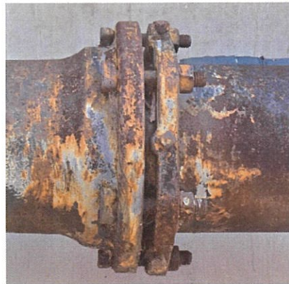
Figure 12: Heavy corrosion at joint
