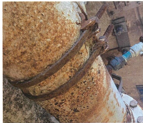
Figure 8: Corrosion on bolt hangers
