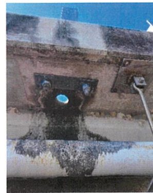
Figure 2: Bridge scupper draining onto force main
