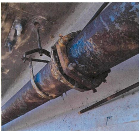
Figure 9: Heavy corrosion along water main
