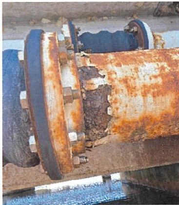
Figure 5: Visible corrosion and coating flaking visible on fire main
