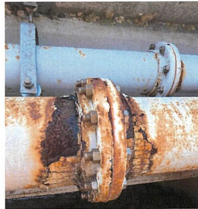
Figure 6: Further corrosion at fitting
