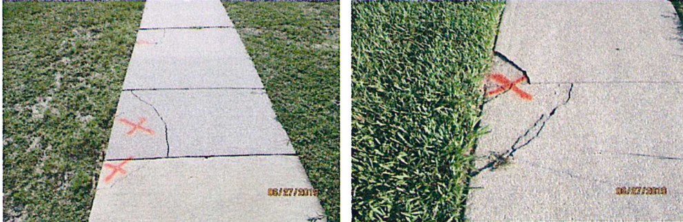
All Repair Areas have been marked with X's
