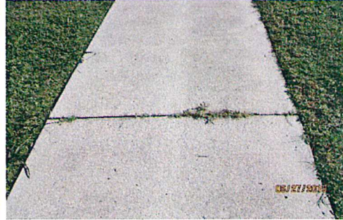
Weeds within Sidewalk Panels
